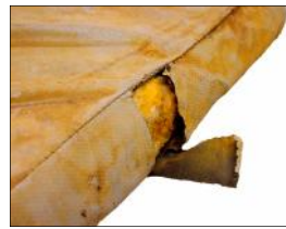
Examples of a corroded fiberglass-reinforced insulation jacketing pad.
